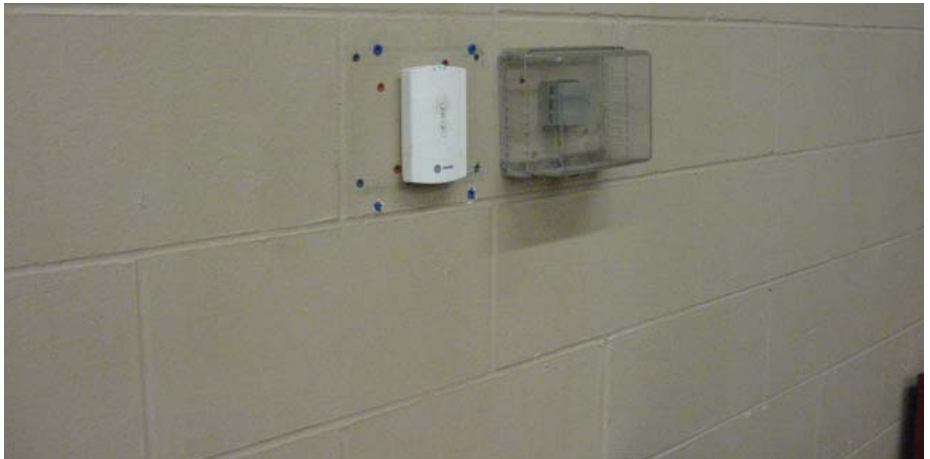
New heat controls to monitor and improve energy efficiency.
